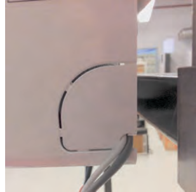
Figure 63: Indoor Unit Knockout (Communication Wires)
