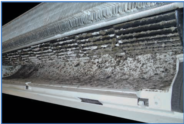
Mini-Split blower with MOLD
