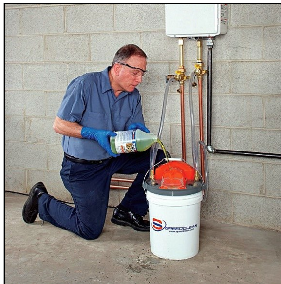
Local plumber descaling and flushing out a tankless water heater system costing both time and money.
